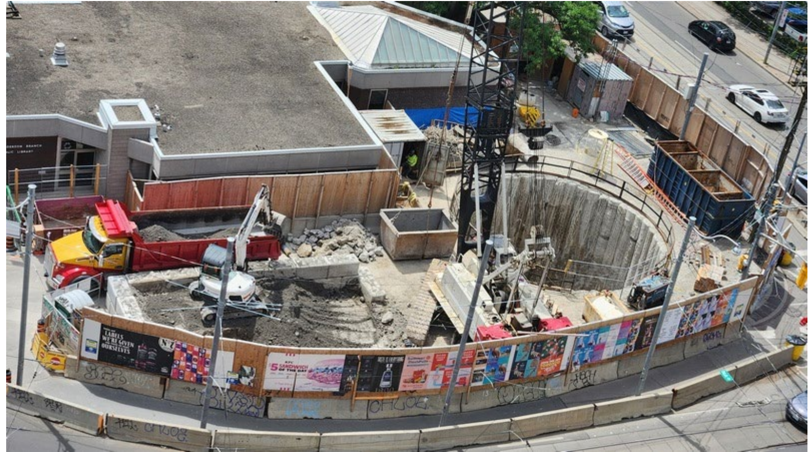
Construction of the Wetwell, where wastewater will be accessed, on the south side of Dundas St. across from TWH.
